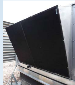
PreVent filters installed on these 40-ton Carrier rooftop units eliminated the need for frequent, extensive chemical cleaning in a Colorado town subject to intense cottonwood seedling invasions.
